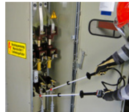
Test with HS 11 at 10 kV transformer
