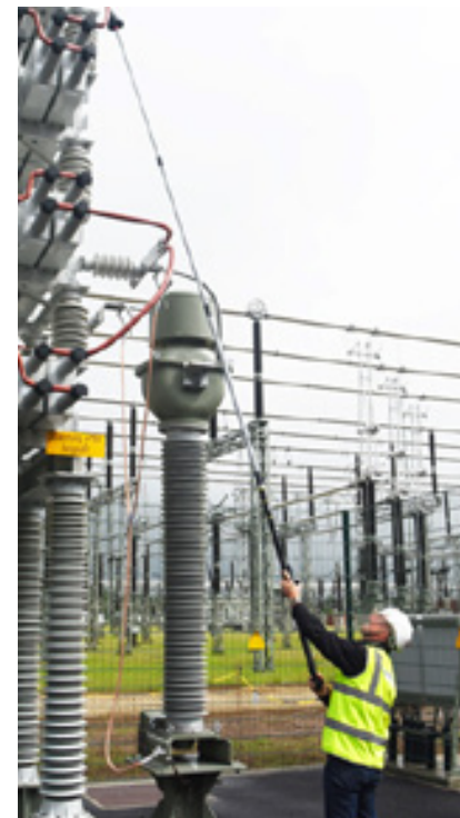
Test at a 36 kV compensation system
